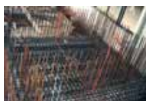
Installation of armouring elements and static armouring elements is performed at the same time
