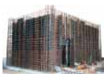
Armouring elements and static armouring elements of a secure room, prepared for panelling and filling with concrete mixture
